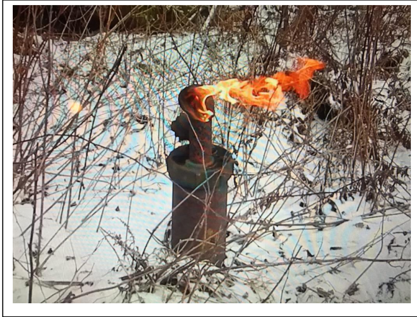
PA Orphan Well emitting unchecked methane (methane lit in order to depict)
